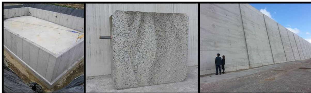
Fig. 1. Kubik building foundation and basement walls (left); a concrete block from the Punta Lucero dock (center) and the Punta Sollana dock wall (right), both at Bilbao Harbor (Spain).
