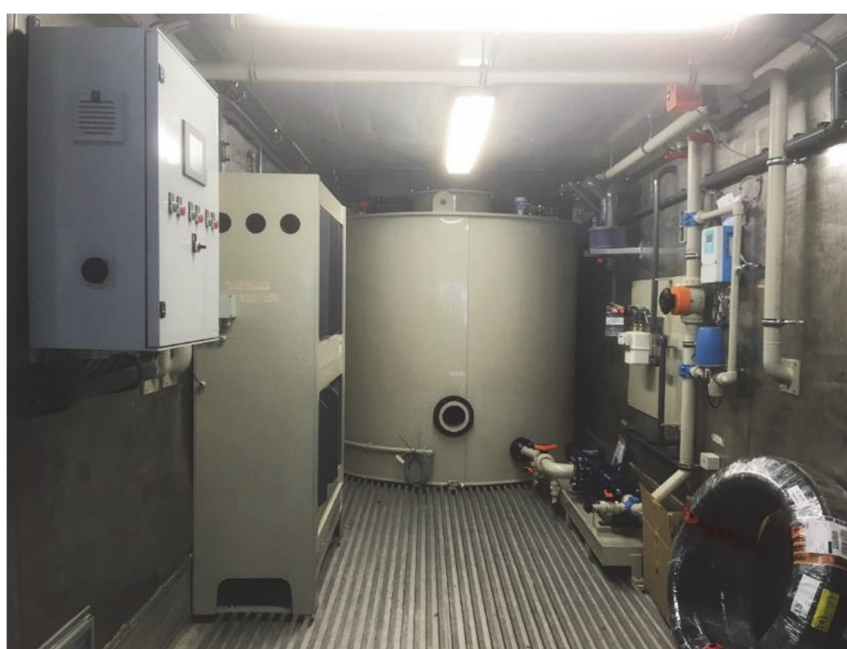
Figure 7: The VOLATILE pilot VFA production reactor
